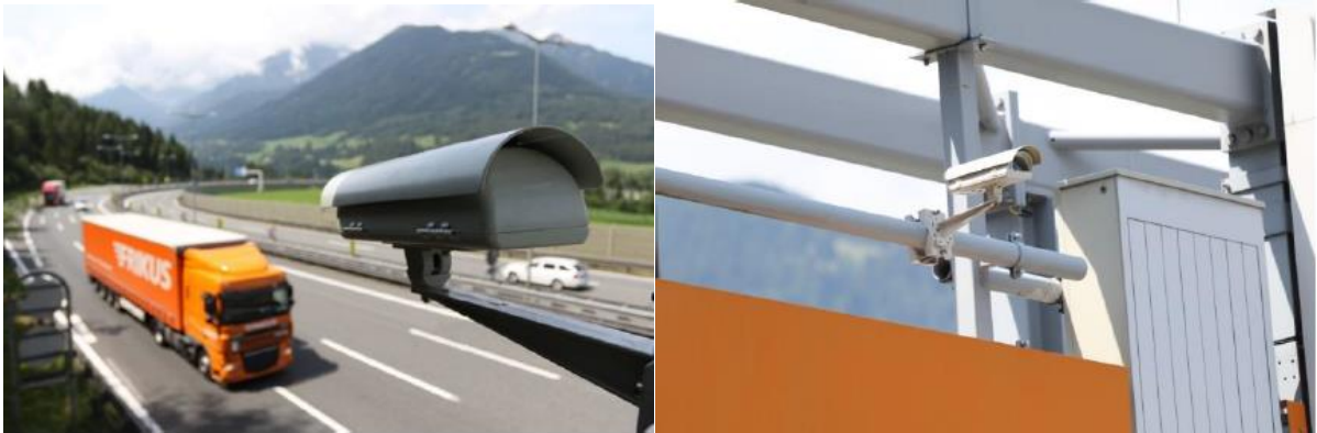
Abbildung 4: System 1 – Maut-Gantry (links); System 2 – Maut-Gantry (rechts)
